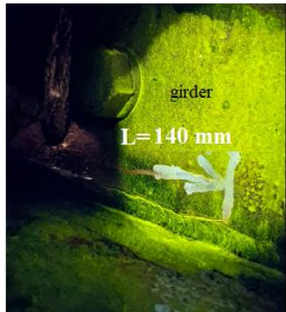
Fig. 4 A fatigue crack in the heat affected zone of a steel girder under an orthotropic plate
